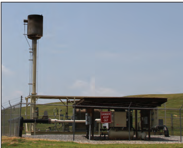
Methane Flare Station
